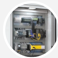
Control panel technology, DIN rail terminal blocks
